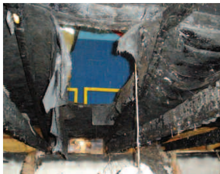
Tests show the deterioration of roof sheathing and the ultimate failure of the roof shingle materials.
